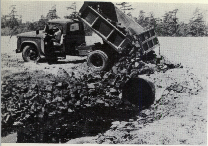
9. Truck loads of broken up asphalt were dumped around the exhaust side of the spillway, and also hand-placed down-stream from the drain to prevent erosion
