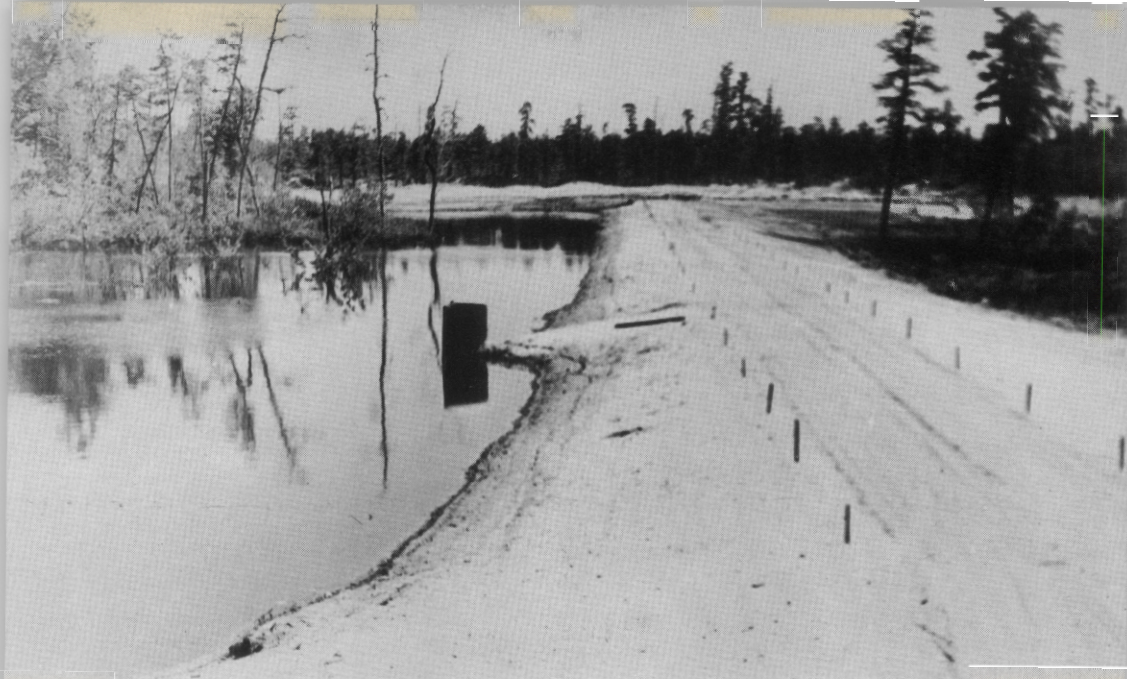
12. The final product. A dike 730 feet long, with a 4 to 1 slope. The dike is 65 feet wide at the base, 9 feet high, and has a 13-foot roadway on top. A total of 11,159 cubic yards of fill was moved to construct the dike. During the winter of 1966, several acres of brush and trees were hand-cut on the pond while it was frozen
