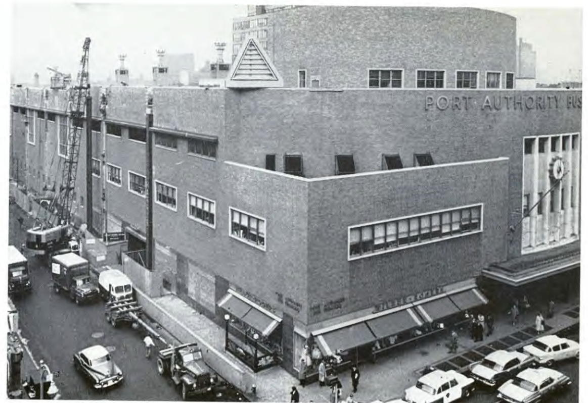
Erection of exterior steel columns to support a new three-level parking superstructure to be built atop the Port Authority Bus Terminal in mid-Manhattan was begun late in the year. The work is a part of the $20,250,000 program to expand suburban and long distance bus operating facilities by 50 per cent. The expansion will be completed in 1962.
