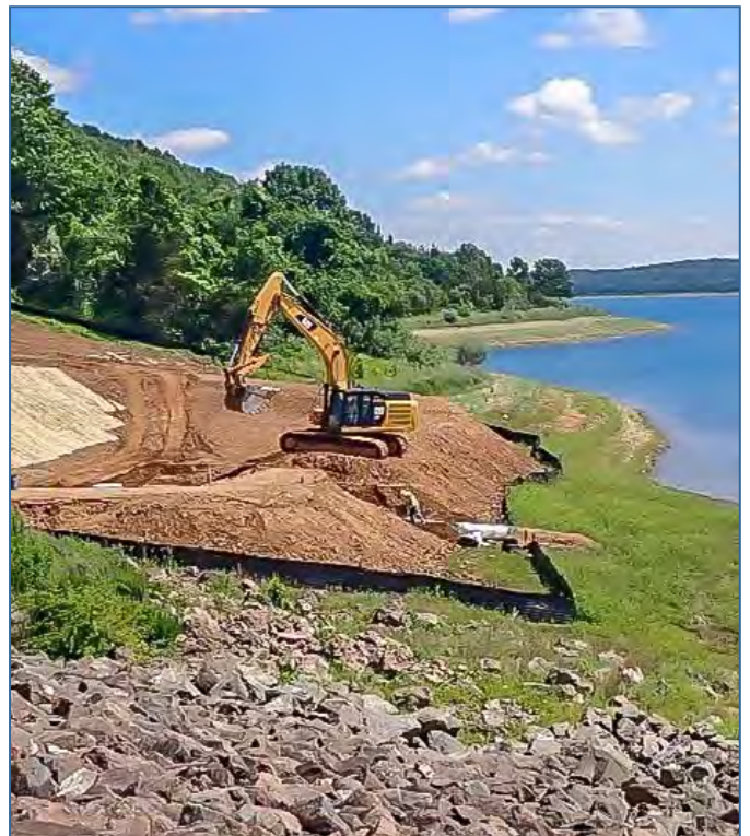
New Jersey Water Supply Authority: Round Valley Reservoir Refurbishment and Resource Preservation. SFY2024 Water Bank Long-Term Loan: $75,000,000
