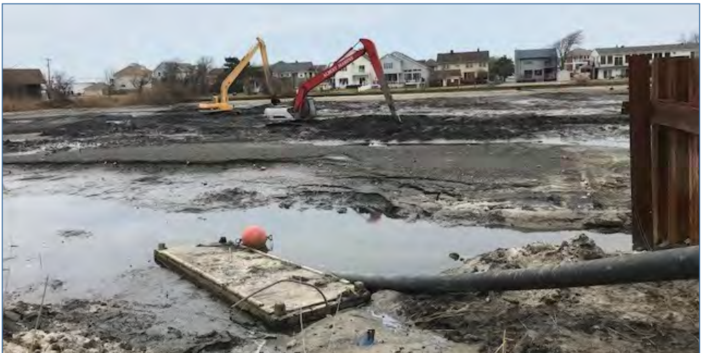
Point Pleasant Beach Borough: Water Main Replacement. SFY2024 Water Bank Long-Term Loan: $2,704,264
