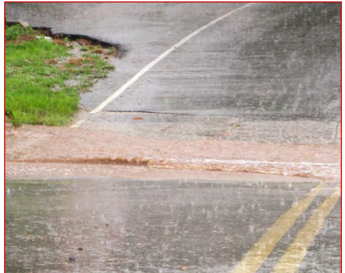
A flooded roadway, underscoring the impact of heavy rainfall and the critical need for resilient stormwater management systems to mitigate such events.
