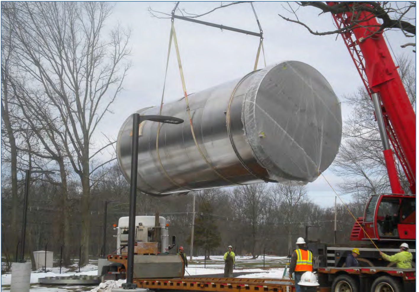
East Orange: Water System Improvement and Resiliency. SFY2024 Water Bank Long-Term Loan: $15,567,005.
