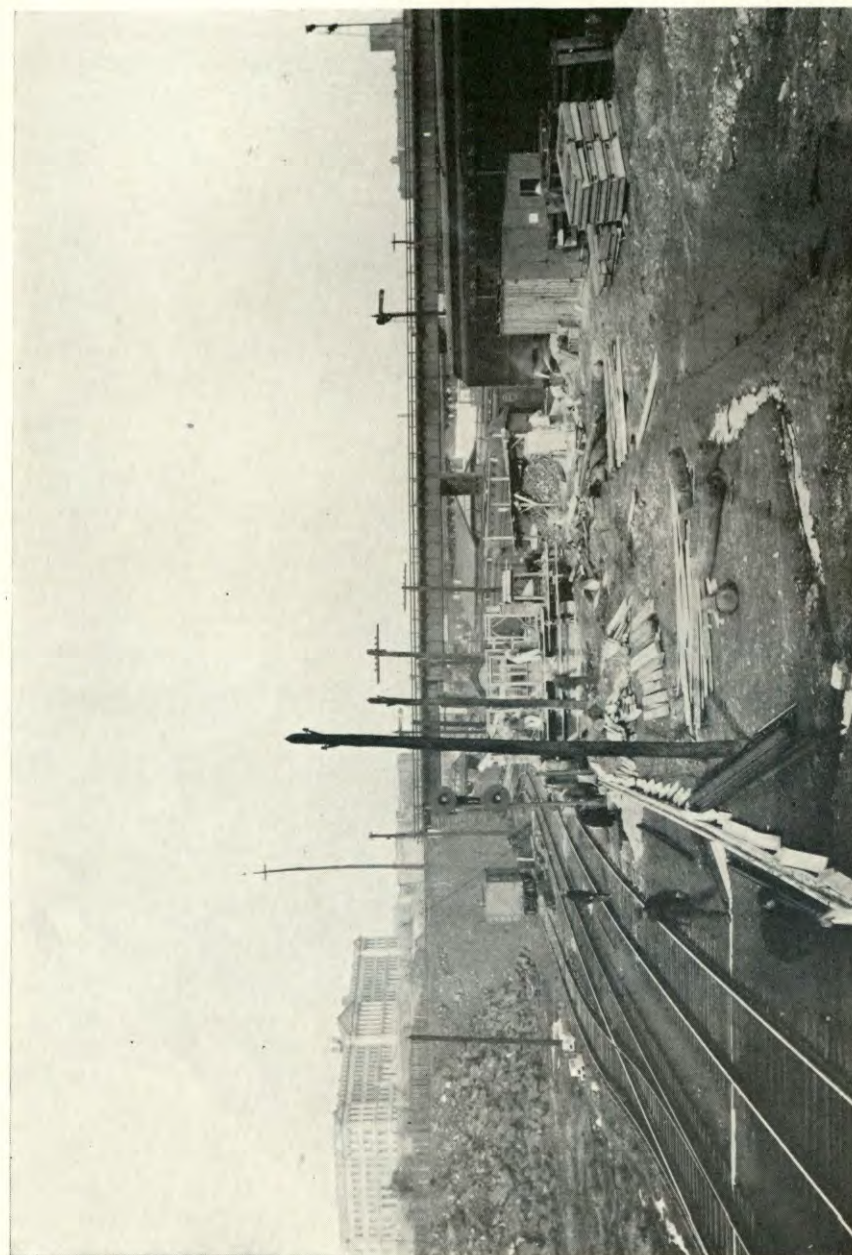
BELT LINE NO. 13 National Junction, showing construction work on new interlocking signal plant for use by Director of Operations.
