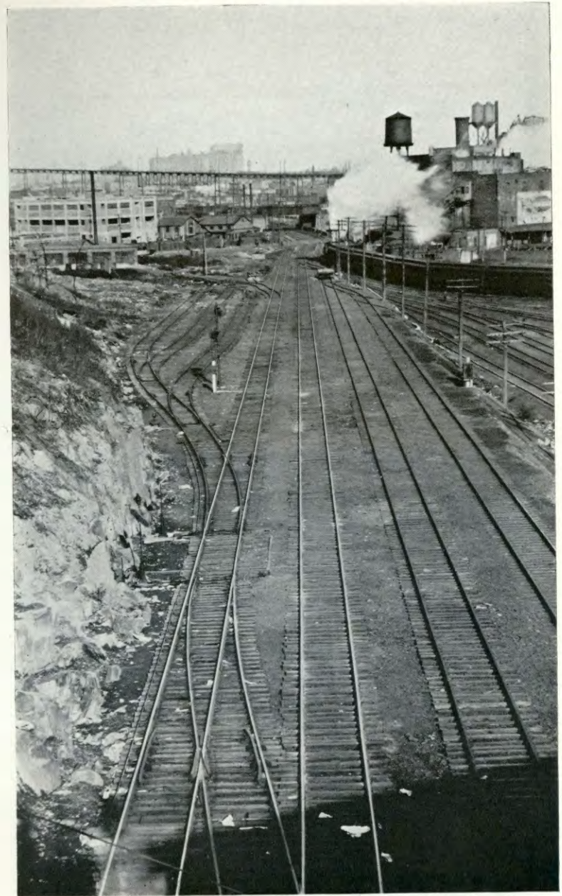
BELT LINE N. 13 View looking north on new construction work for interchange facilities to handle Pennsylvania Railroad business, vicinity of Fifteenth Street, Jersey City.
