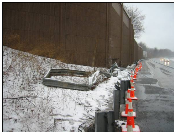
W-Beam Barrier on Interstate 295 Damaged by a Tractor Trailer
