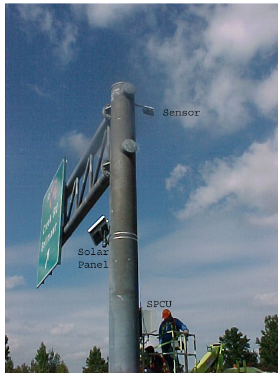
Figure 3. Surveillance System Picture
