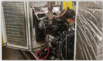
Figure 20: Rutgers University's cogeneration system.
